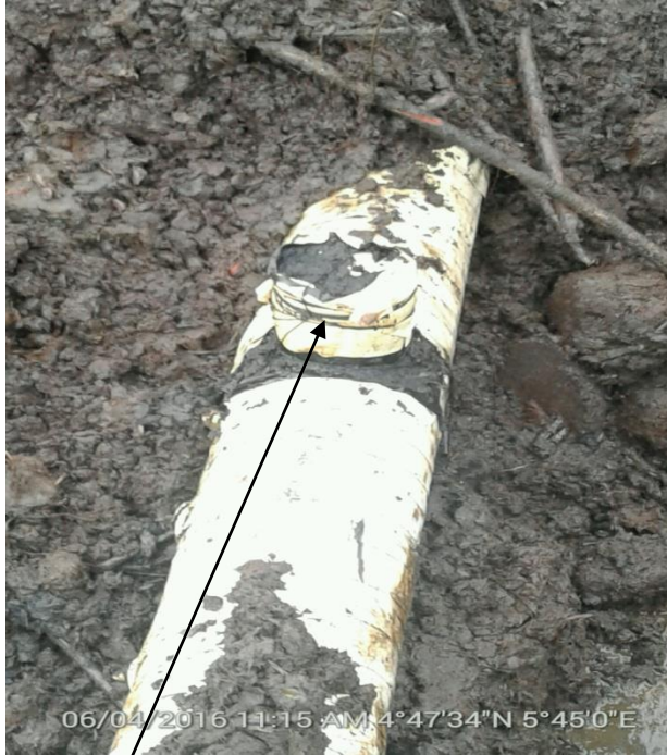
Tampered previously repaired point
