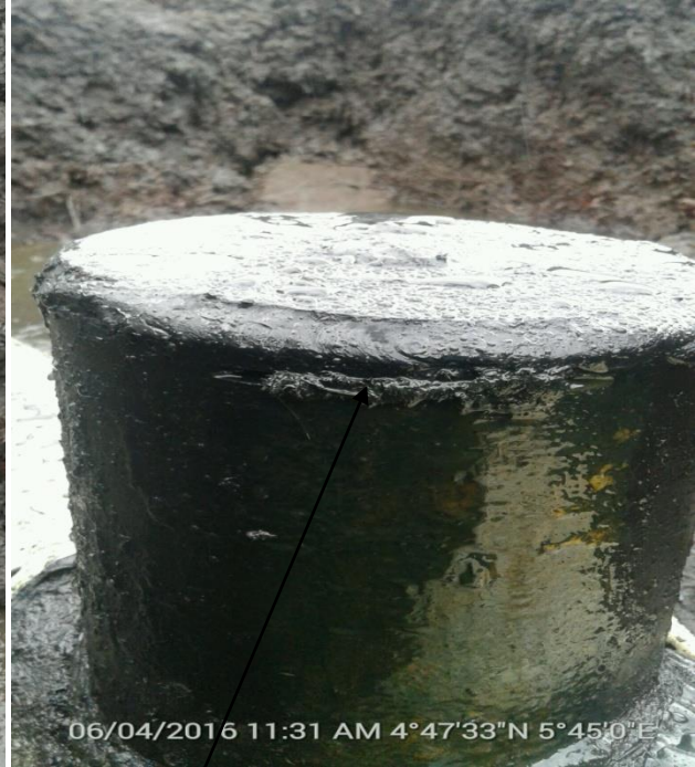
Hacksaw cut on previously repaired point
